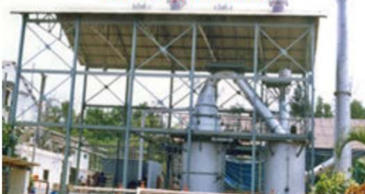
Dual Combined Incenerator
