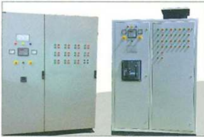
Automatic Harmonic Filter Panel
